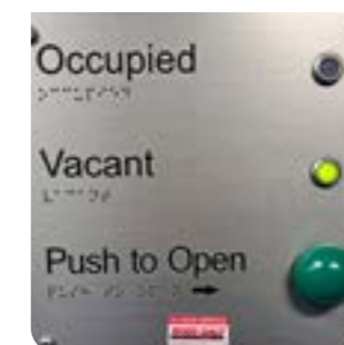
Level 1 accessible toilet entry button
